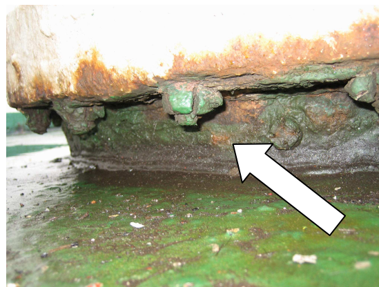
Example of corroded bolts
